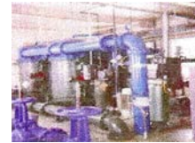
Water Treatment Facility
